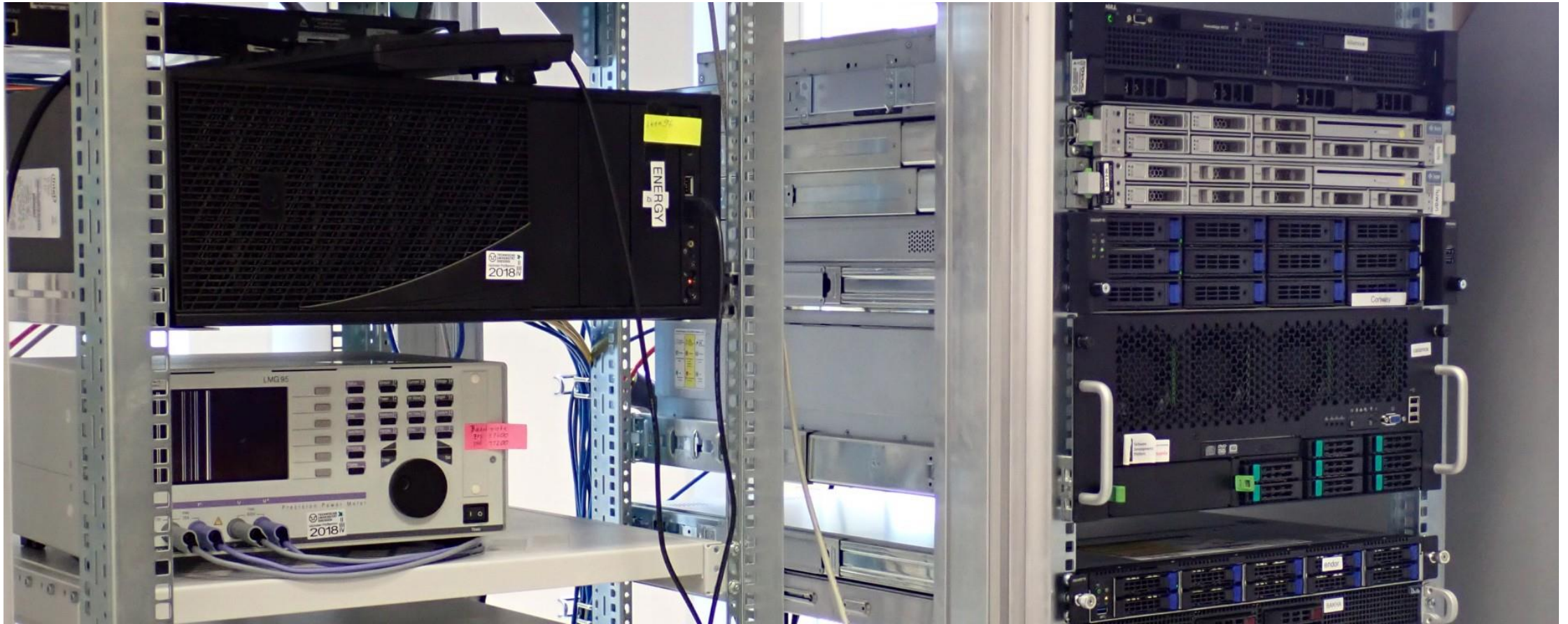
Racks in Energy Lab @ TUD
